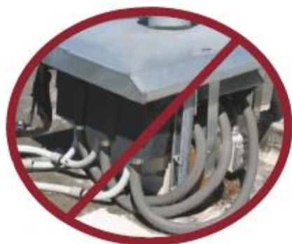
No more leaks with old school Pitch-Pans!
